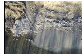
Tara River muddy from the construction site wastewater (Jabuka stream, November 2018)
